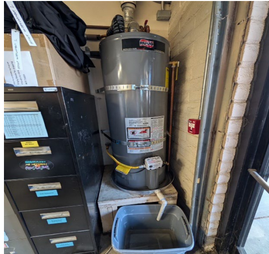
New Water heater
