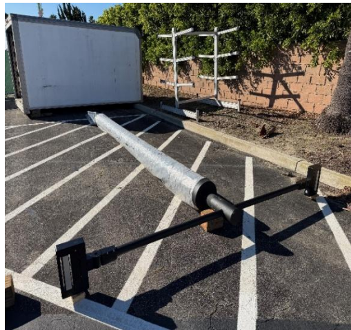
Light head to pole connection
