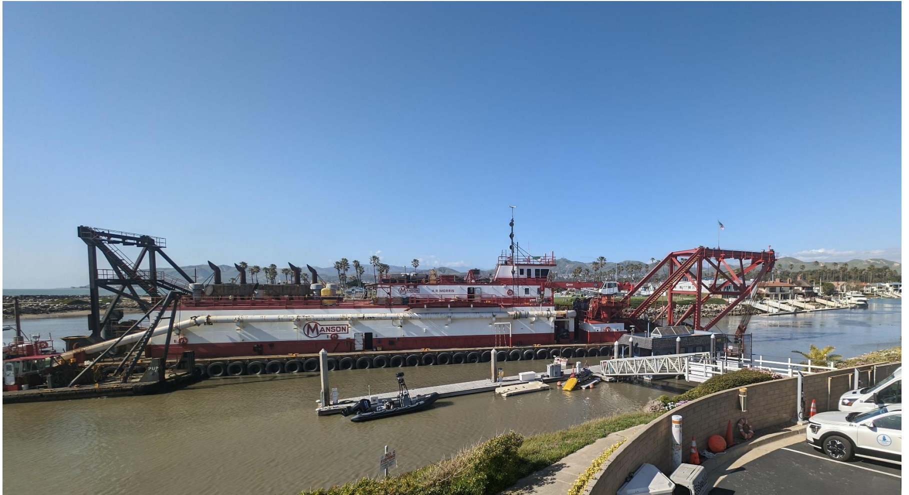
HR Morris dredging the inner harbor “Stub Channel” that connects the Ventura Keys to the harbor entrance.
