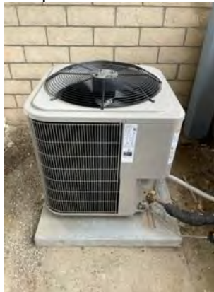
New 5-Ton HVAC compressor
