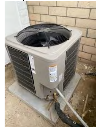
New 5-Ton HVAC compressor
