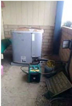
Old Compressor to be removed
