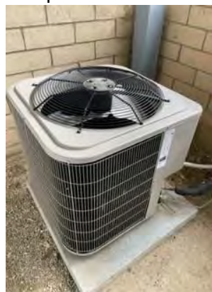
New 5-Ton HVAC compressor
