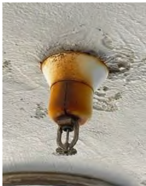
Rusted sprinkler head escutcheon and skirt
