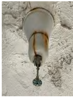
Rusted sprinkler head escutcheon and skirt
