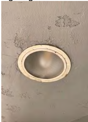
Obsolete outdated Lighting fixture
