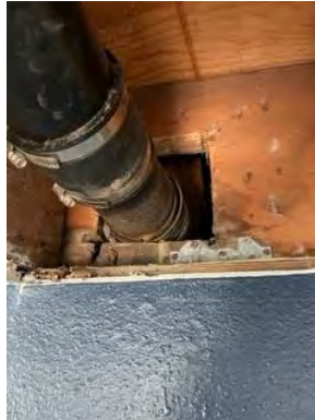
failed cast pipe in soffit
