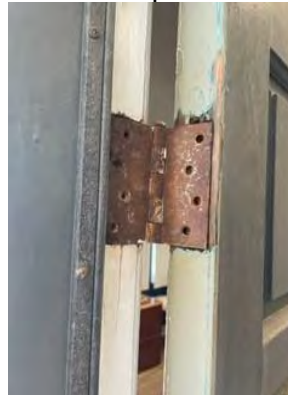
Inner door trim in need of paint
