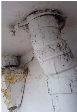
Leaking roof drain
